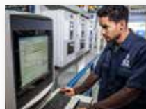
Distributed control platform for control isolation
