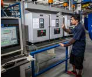
Distributed control platform provides peace of mind for mission critical systems
