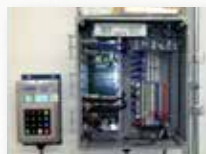
UtiliPulse hardware is used to monitor any customer supplied meters
