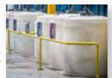
Monitor chemical usage
